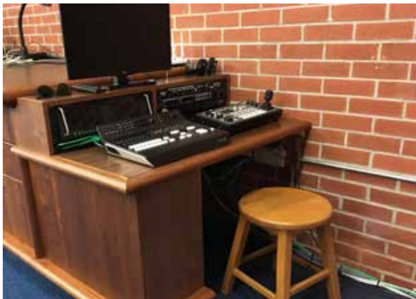
A new video system and cabinetry for San Rafael chamber.
